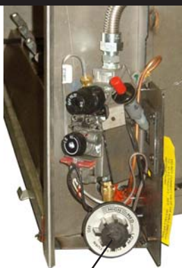
rear burner control knob
