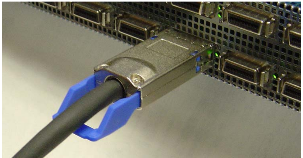
Figure 1-11: Fully Installed IB Cable with Pull Connector
