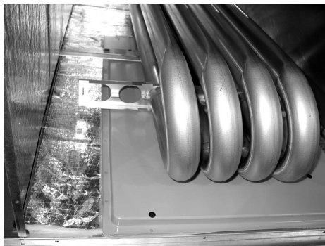
FIGURE 15 - DISCHARGE PANEL IN PLACE
