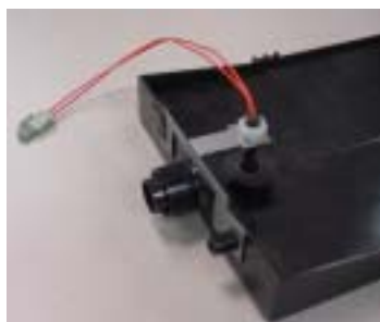
Figure I-MR-1. Condensate float switch installed in horizontal auxiliary drain pan.
