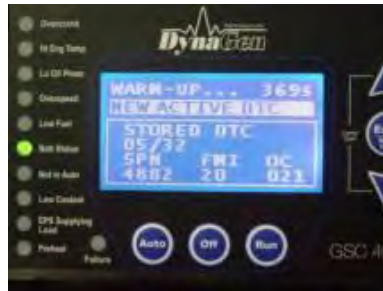
Figure 15 – 32 stored DTC messages, the 5PthP stored code being displayed
