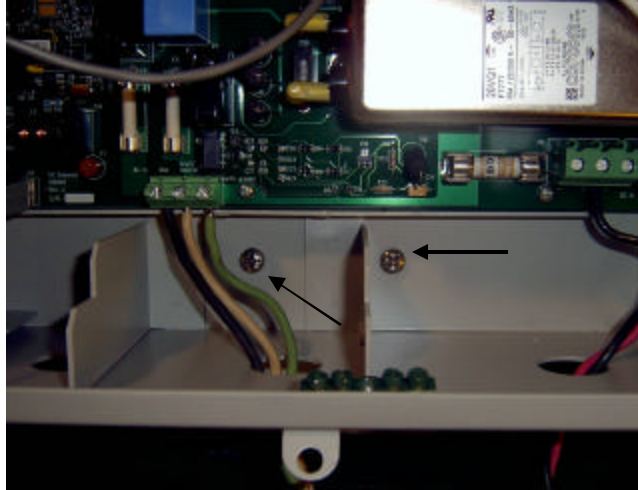
Figure 3: Inside screws, located below the power board
