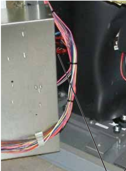
Figure 13A: Wire access (control box open)
