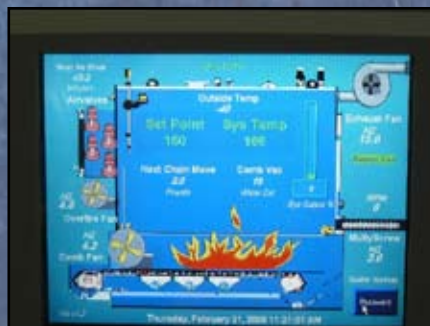
Touch Pad Control Panel
