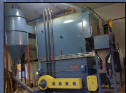
10,000,000 BTU Hot Water Boiler heating a greenhouse
