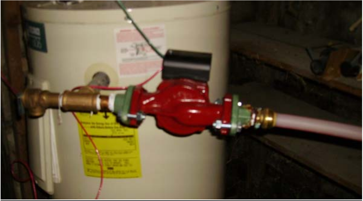
Customer supplied photograph: Make sure using a single wire is to code in your area.
