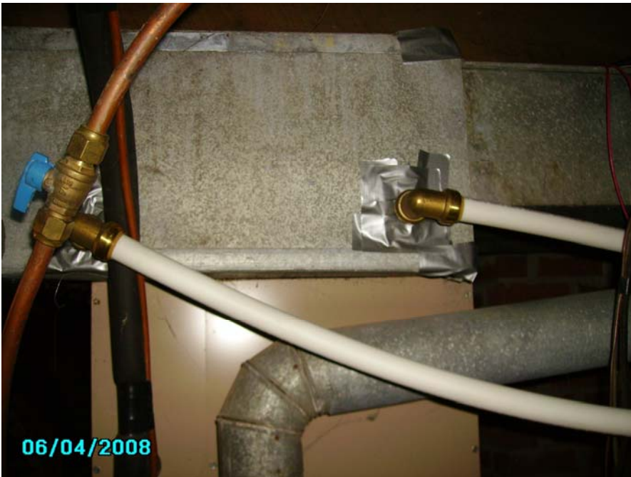
A customer's photo of his heat exchanger installation.
