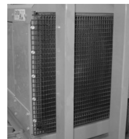
RADIATOR SCREEN - CLEAN FROM THIS SIDE
