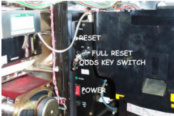
RESET SWITCH ON INSIDE OF DOOR
