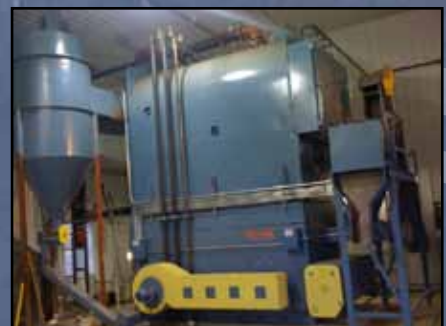
10,000,000 BTU Hot Water Boiler heating a greenhouse
