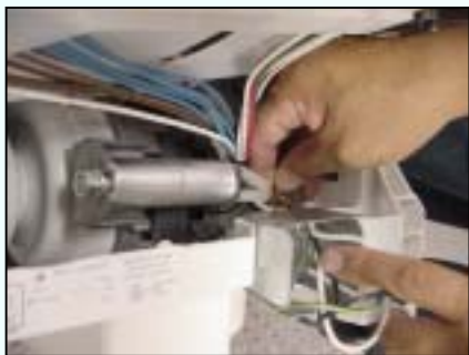
Pull wires from J-box
