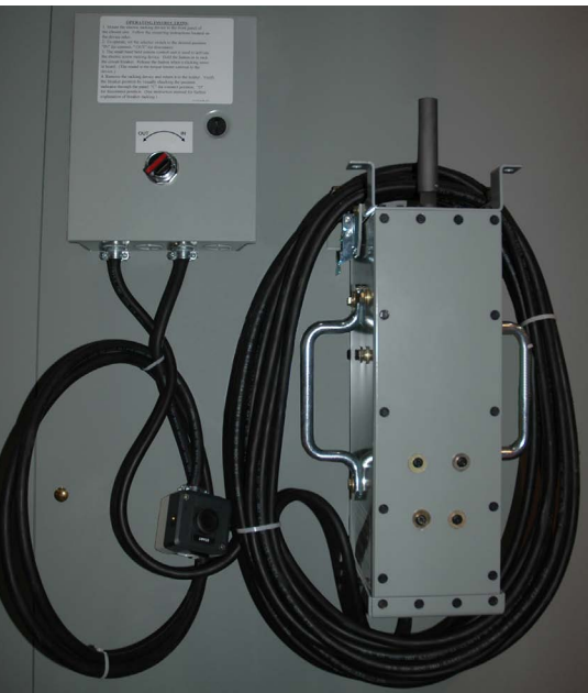
Figure 5: Electrical racking accessory mounted on the switchgear
