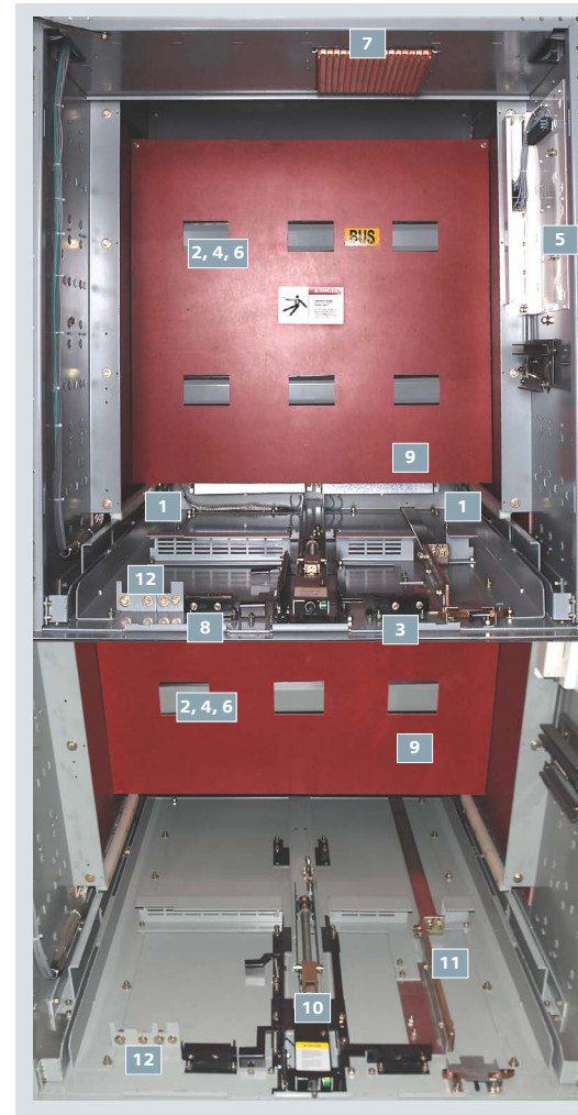
Figure 3: Two views of same circuit breaker cell interior
