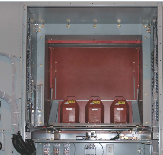
Figure 8: VT cell with fuse truck withdrawn (shutter closed, VT primaries grounded)
