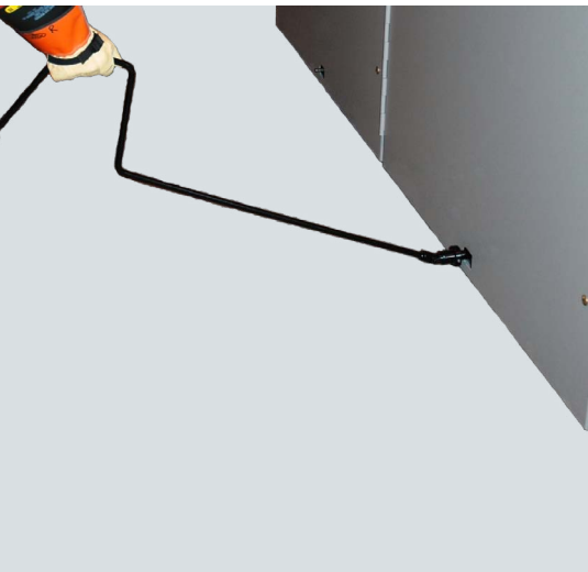
Figure 4: Circuit breaker being racked out with door closed
