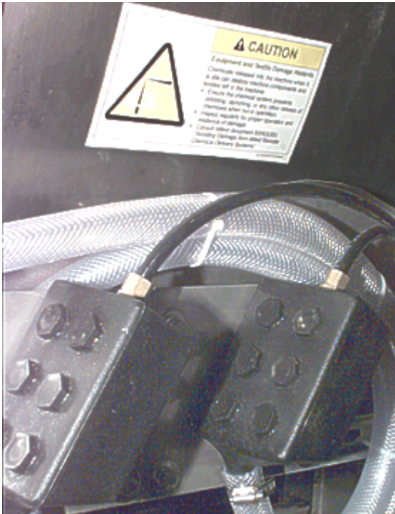
Figure 1: Pumped Chemical Inlets on CBW Batch Washer
