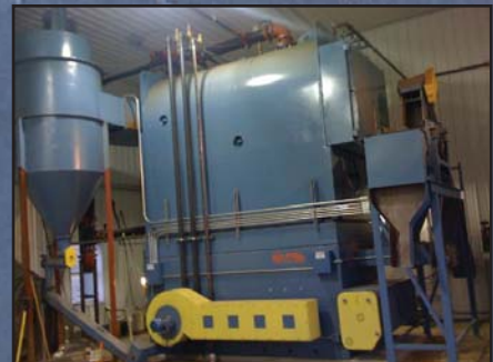
10,000,000 BTU Hot Water Boiler heating a greenhouse
