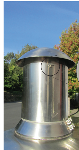
Flue collapsed and locked.
