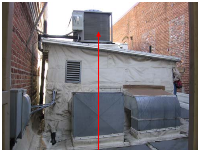
Heat Pump #4 on shed roof (Large air handler is inside shed)
