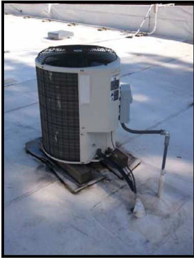
1.5 Ton Heat Pump on Roof
