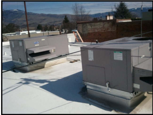
Two 4 Ton Heat Pumps on roof
