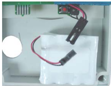
Figure 10-4 – Removing the Used Battery Pack
