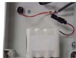
Figure 8-6 – WPR Battery Pack Connected
