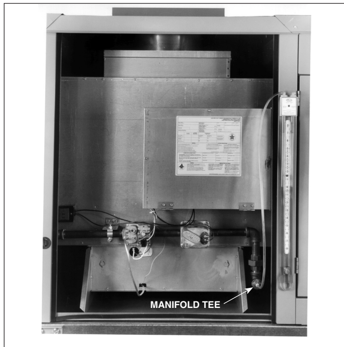
Figure 9.1 Checking Manifold Pressure with “U” Tube Manometer
