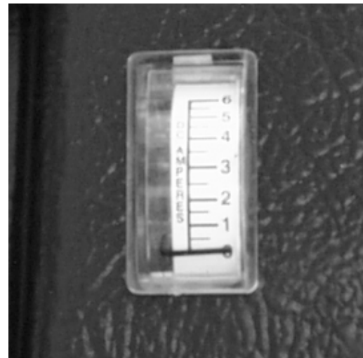
Figure 11. Ammeter Indicates Battery Is Fully Charged
