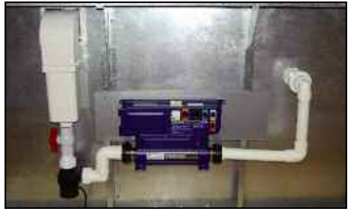
Completed water quality system.
