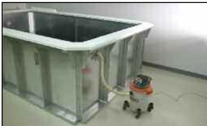
Vacuum in place before liner is hung. Note thru-wall holes are sealed.
