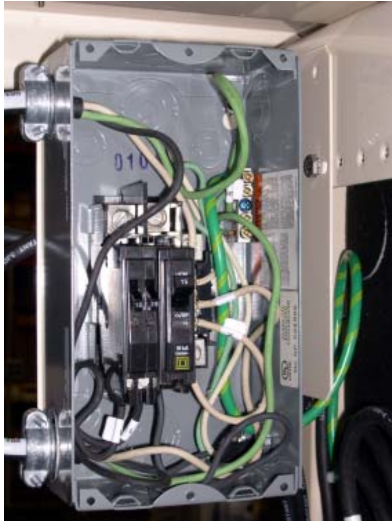
Fig. 3-8, Service Power Breaker box (RMB-E-911-B)
