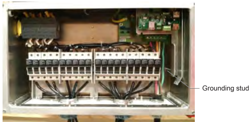
Figure 4-5. Grounding stud in the connection box
