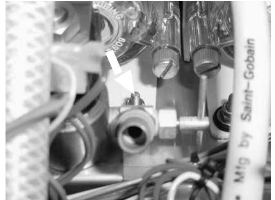
FIG 8 Chilled Water Flow Valve P3487
