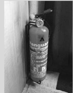
Fitted Fire Extinguisher in situ
