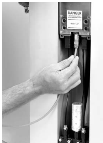
Connecting the PC to the controller
