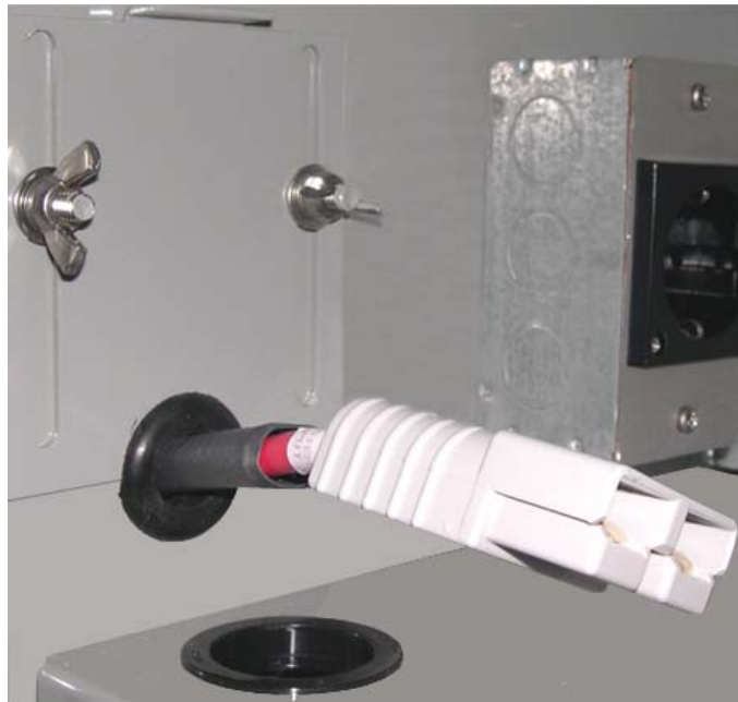
Fig. 3-1, Generator Access Door and Battery Pack Adapter Cable
