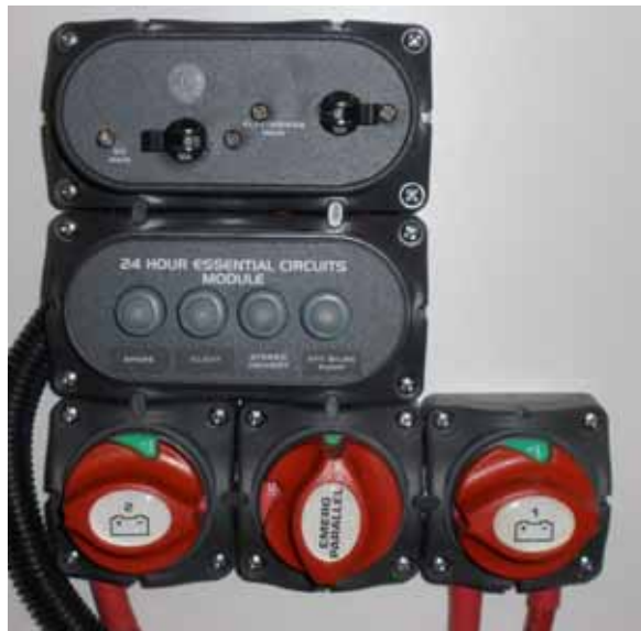
Battery Switches and Main Breakers
