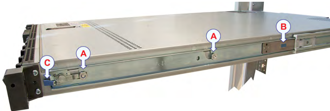
Figure 29 TRC Beamformer computer installation
