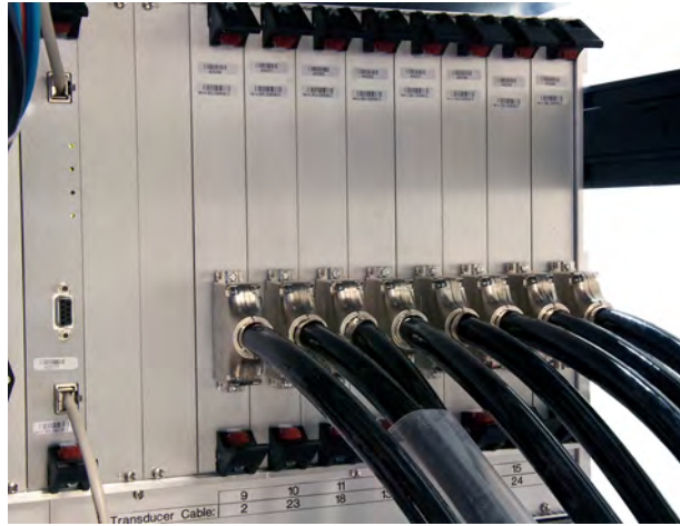
Figure 33 Transducer cables connected to the rear side of the TRXU rack
