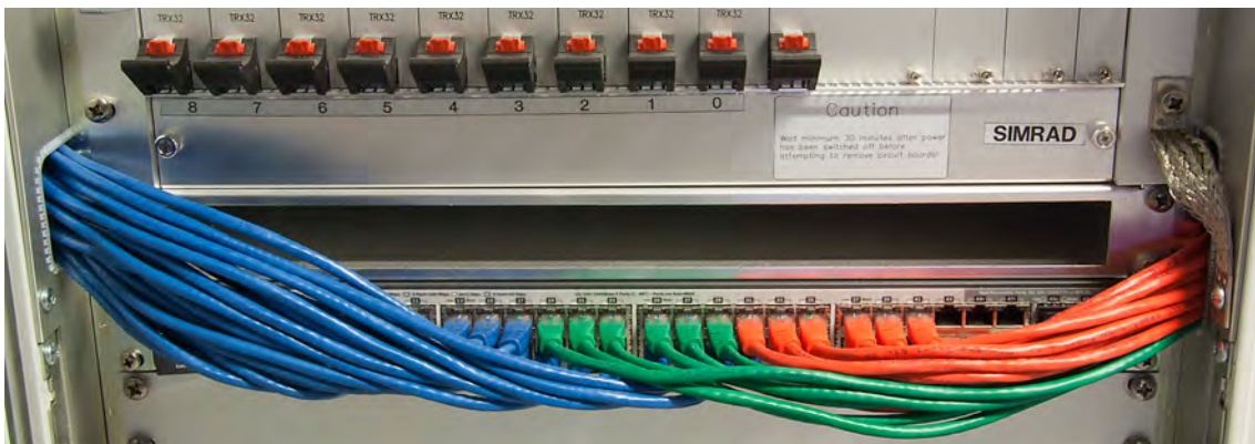
Figure 28 Ethernet switch with all cables connected
