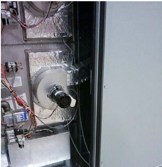
Figure D9: Drain line from flue box to exterior of casing
