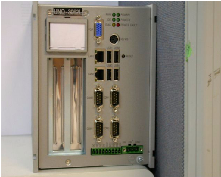
Figure 3.7: UNO-3072L Improper Installation (2)
