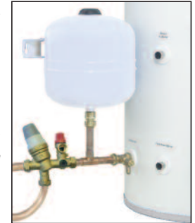
Inlet group with expansion vessel position (Tempest only) also shows drain off position and balanced supply.
