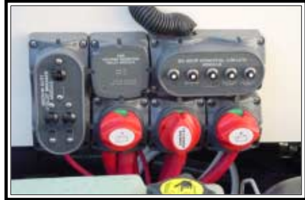
Battery Switch Panel
