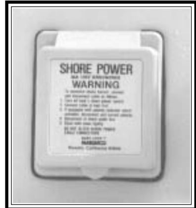
Shore Power Inlet
