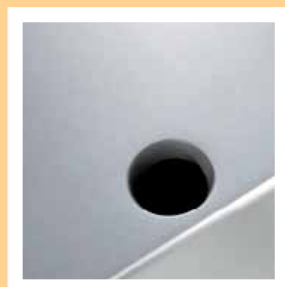
Large drain hole
