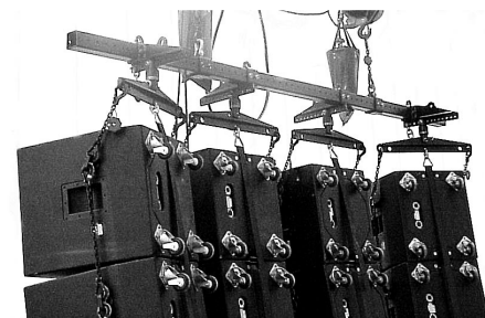
Rear view of the top row of a 4-wide Installer flying system
