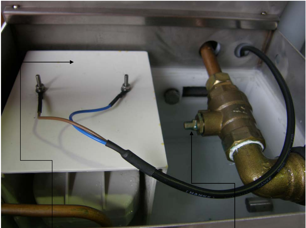
Ball float adjustment under Water flow regulator valve
