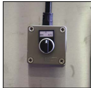
Manual Off/Auto switch install on ITS
