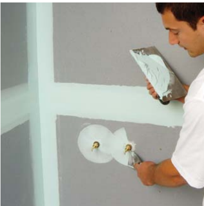
4. Apply skim coat of Wet Area Taping Cement at joints and around penetrations.
