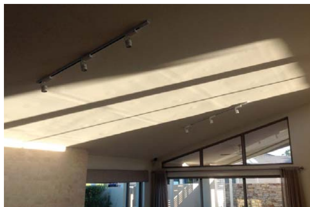
Figure 7: Same plasterboard surface under glancing light
