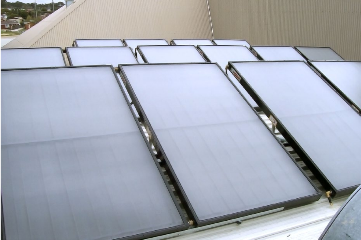
Figure 13. Solar collector array installed on a flat roof
