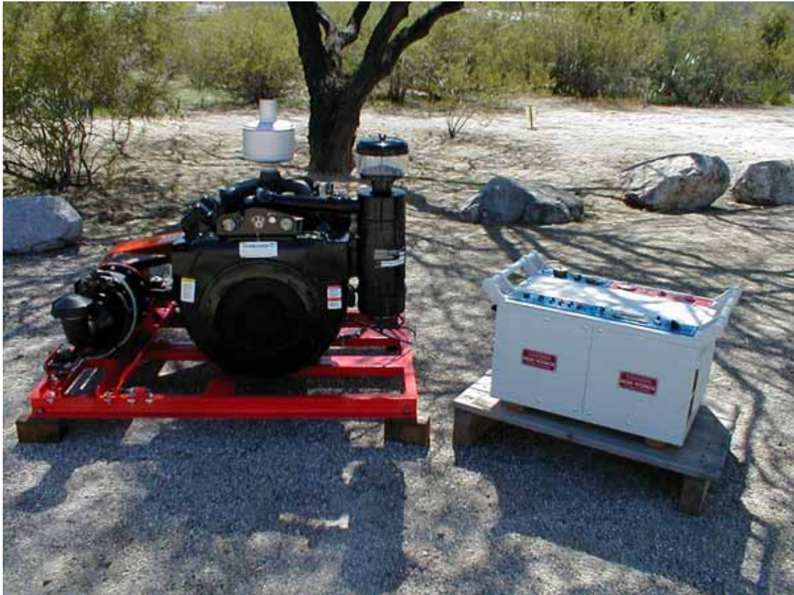
Figure 4 Motor-Generator Set ZMG-30
