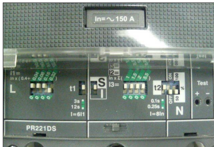
Figure 11 The Dip switch on the breaker CB1
