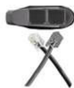
Wrong Wiring but Functional
