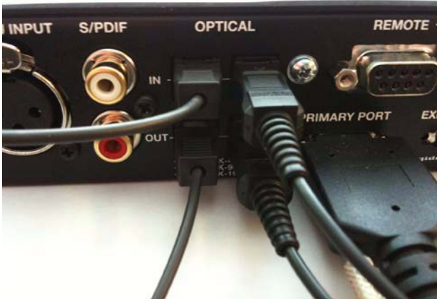
Figure 4. Optical loop back connections
