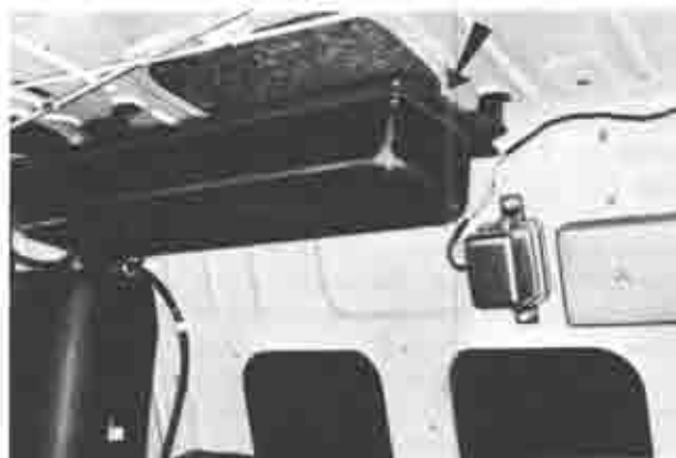
Fig. 1A-30 Condense tank
