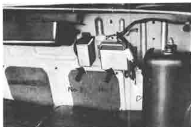
Fig. 1A-19 No. 1 and No. 2 control boxes
