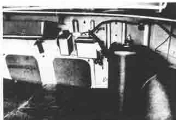
Fig. 1A-37 Condense tank
