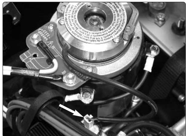
The magnetic brake's electrical connection
