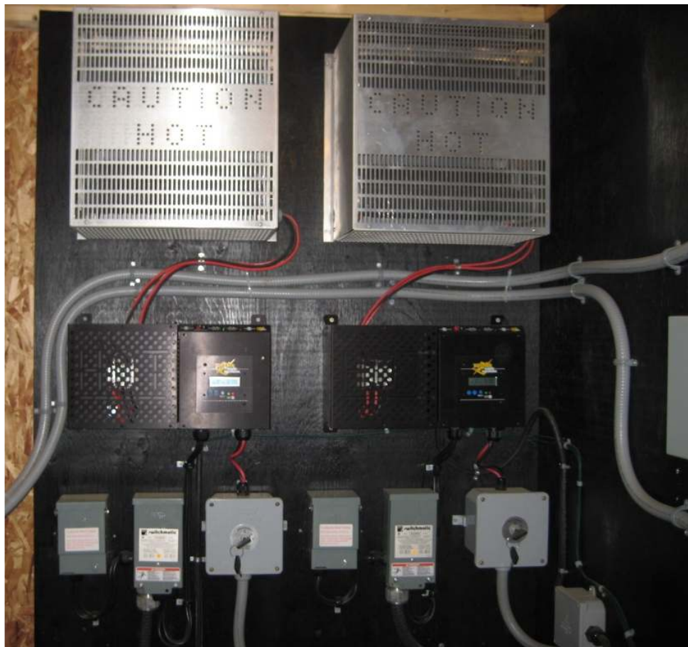
Figure 3: Charge controllers for wind turbines (diversion resistors on top, on bottom; brake, diversion switch, and battery key switch)
