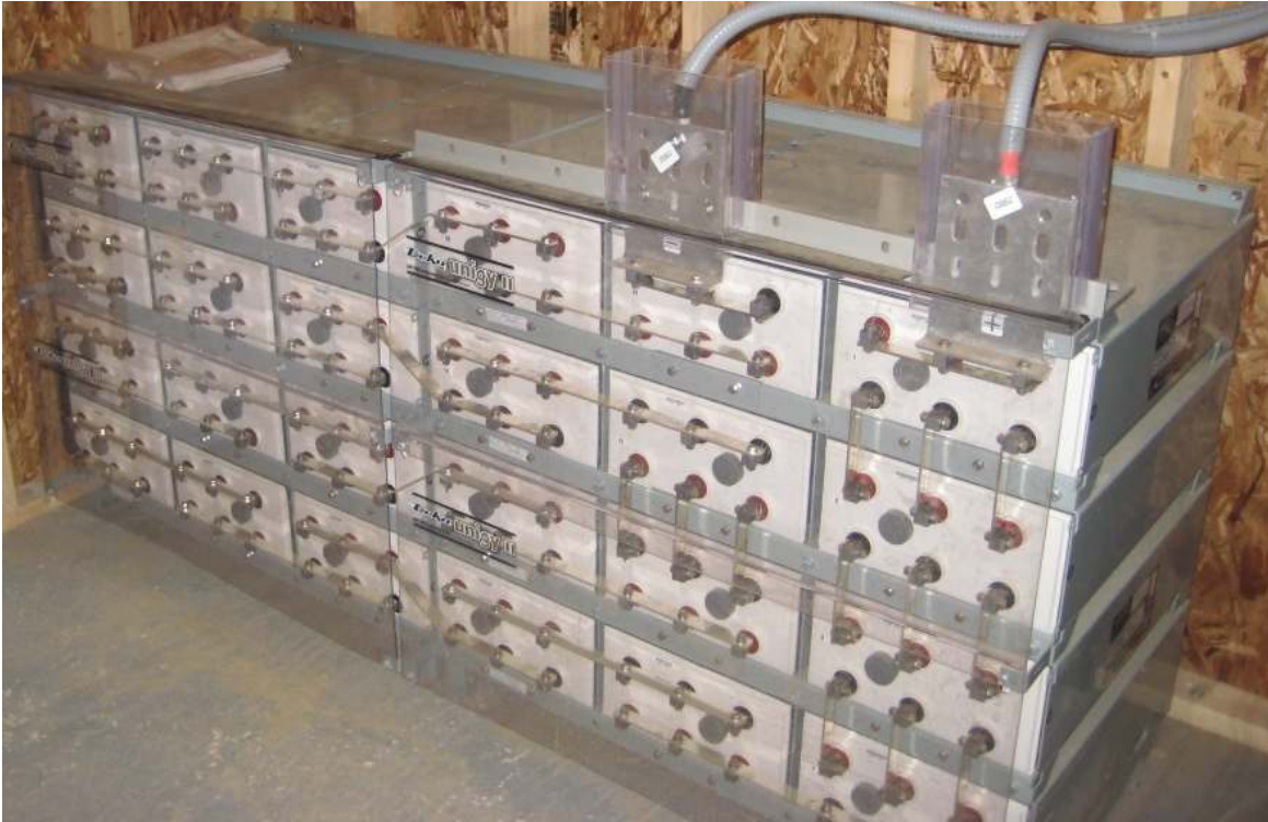
Figure 4: One of three 24 cell batteries – Battery A
