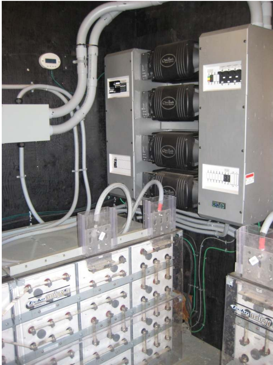
Figure 6: Outback Inverter/Charger system (AC panel on left, DC on right)
