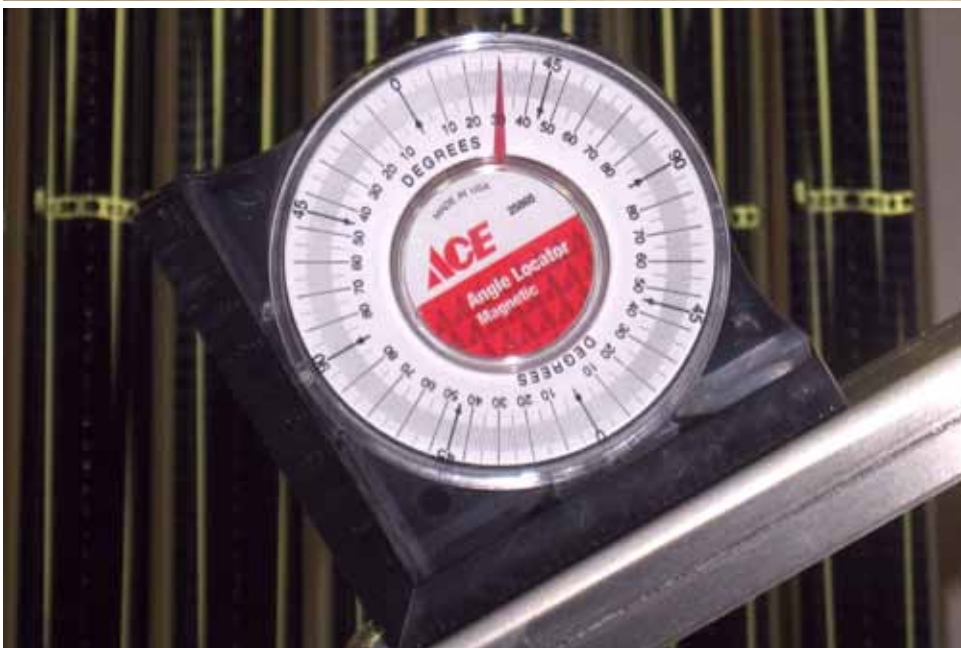
Step 28a: Measure the angle of the assembly to make sure that it is at the required angle. If it is not, then it is necessary to adjust the riser struts. The illustrated assembly is adjusted to 30°.
