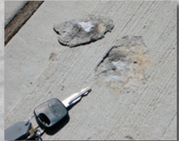
Popout surface damage caused by the fracture of a soft aggregate particle during winter freeze/thaw cycles
