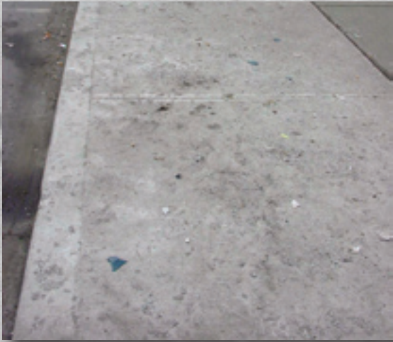
Light scaling of a concrete sidewalk
