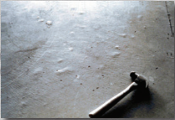
Blistering concrete surface
