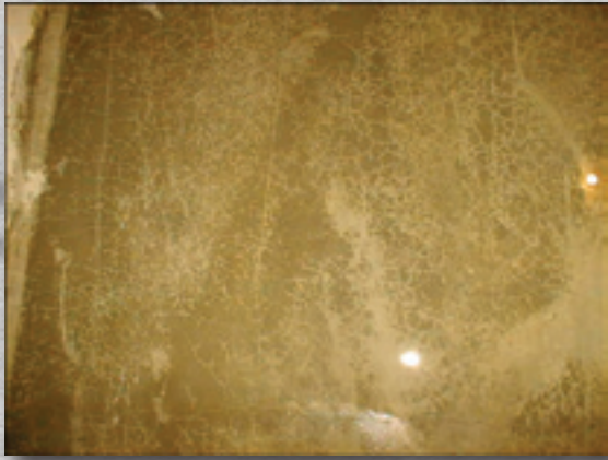
Crazing on a residential garage floor slab
