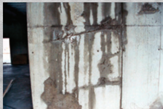
Honeycombing in a residential shear wall
