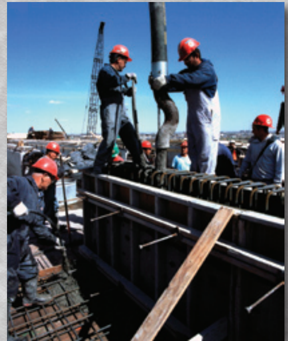
Concrete pumping on a commercial project using a flow restriction device to provide resistance to flow and to prevent direct free fall
