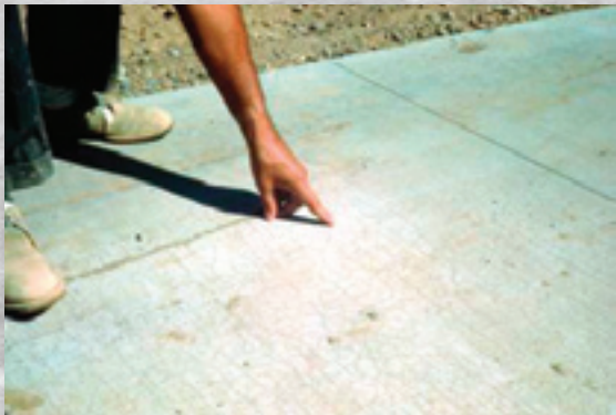
Crazing on exterior flatwork
