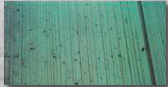
Bugholes on a concrete surface created with a form liner
