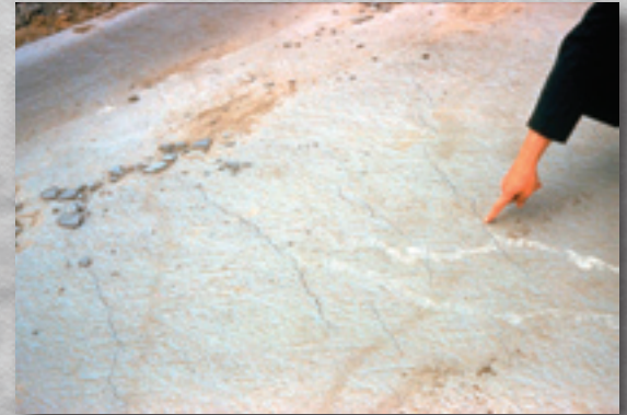
Plastic shrinkage cracks on exterior flatwork
