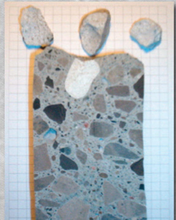
A cross-sectional view of a concrete core taken from a popout area – note the large chert particle in this limestone aggregate source that is responsible for the popout
