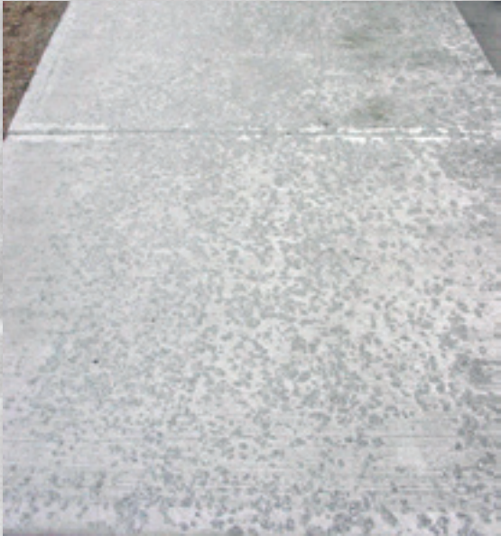
Medium scaling of a concrete sidewalk
