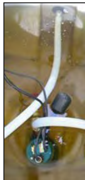
Barnes Submersible Pump in Surge/Pump Tank
