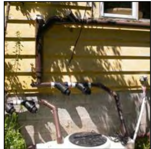
Cleanout on horizontal pipe, high capacity 4" debris filter, and two 2" Y Strainers.
