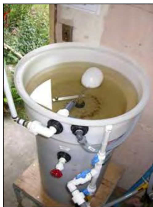
Ball cock valve controls flow into BioSand filter
