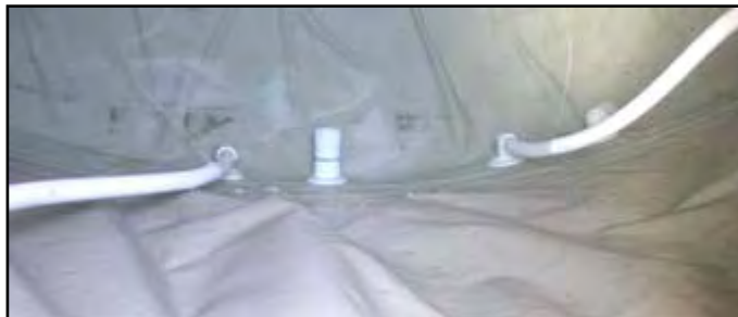
Interior cistern fittings
