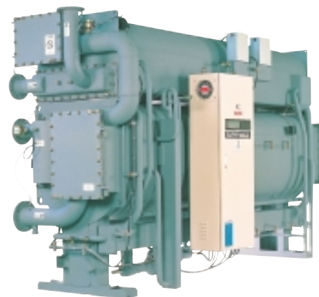
Hot water-fired chillers
